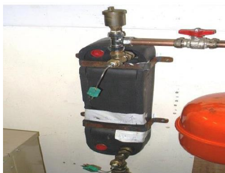
Fig. 14. The heat exchanger.
