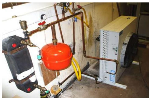
Fig. 15. Shows the connections of the heat exchanger, water pump, heat rejection fan and expansion valve.
